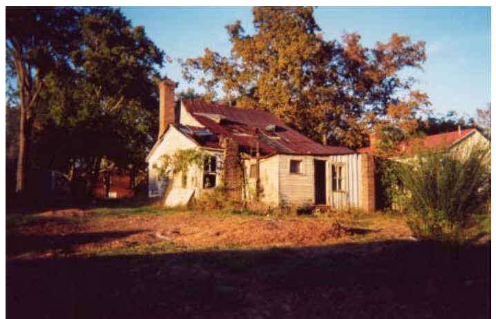
Top and Above: This historic house had been altered numerous times in the past—including multiple additions to the rear of the building.
