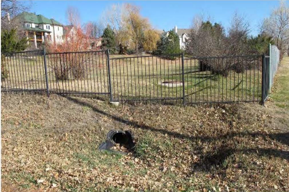
Detention pond viewing east from Mail Creek Drive / pond outfall pipe in foreground
